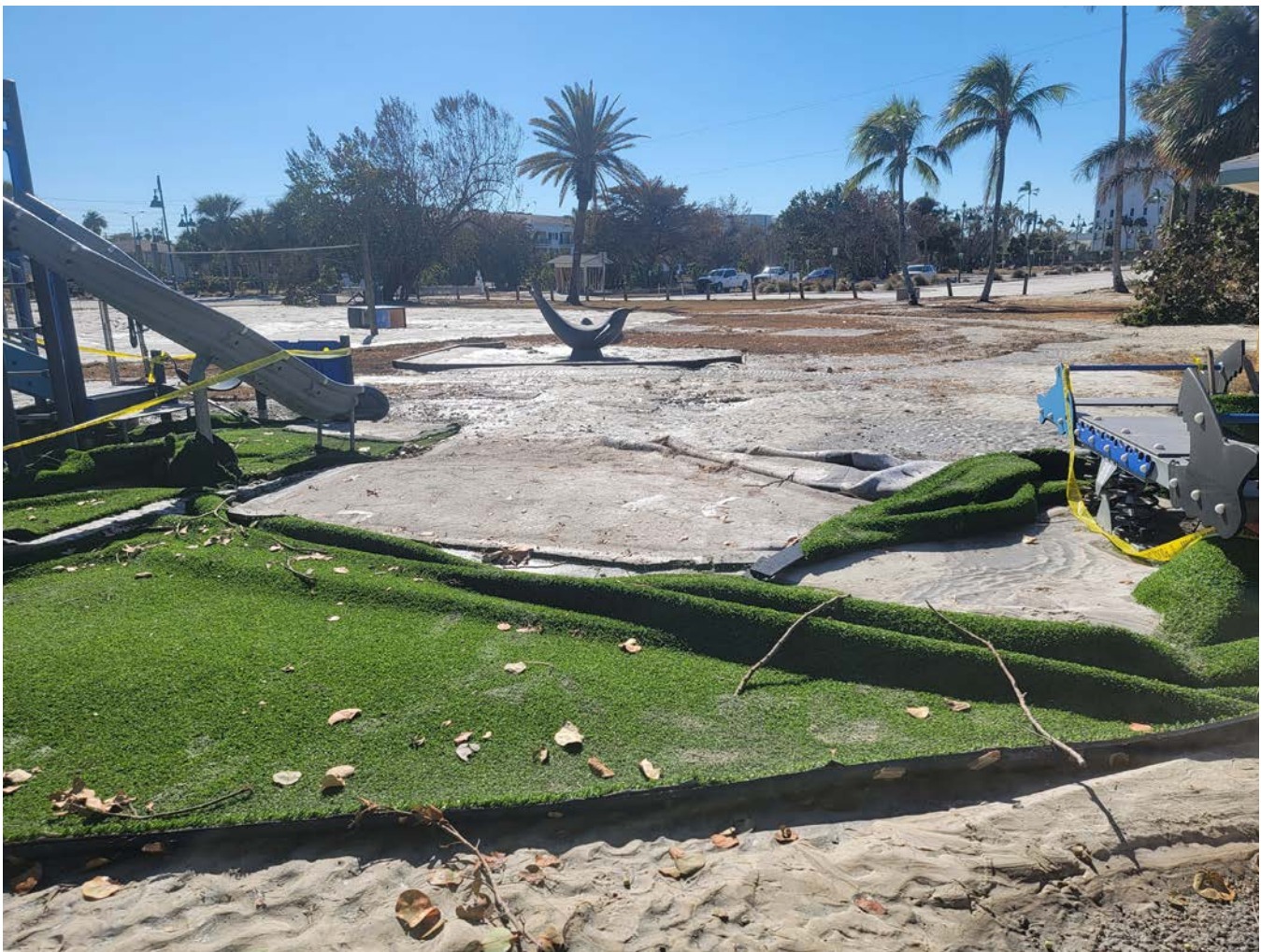
Storm damage at Lowdermilk Beach Park after Hurricane Ian
