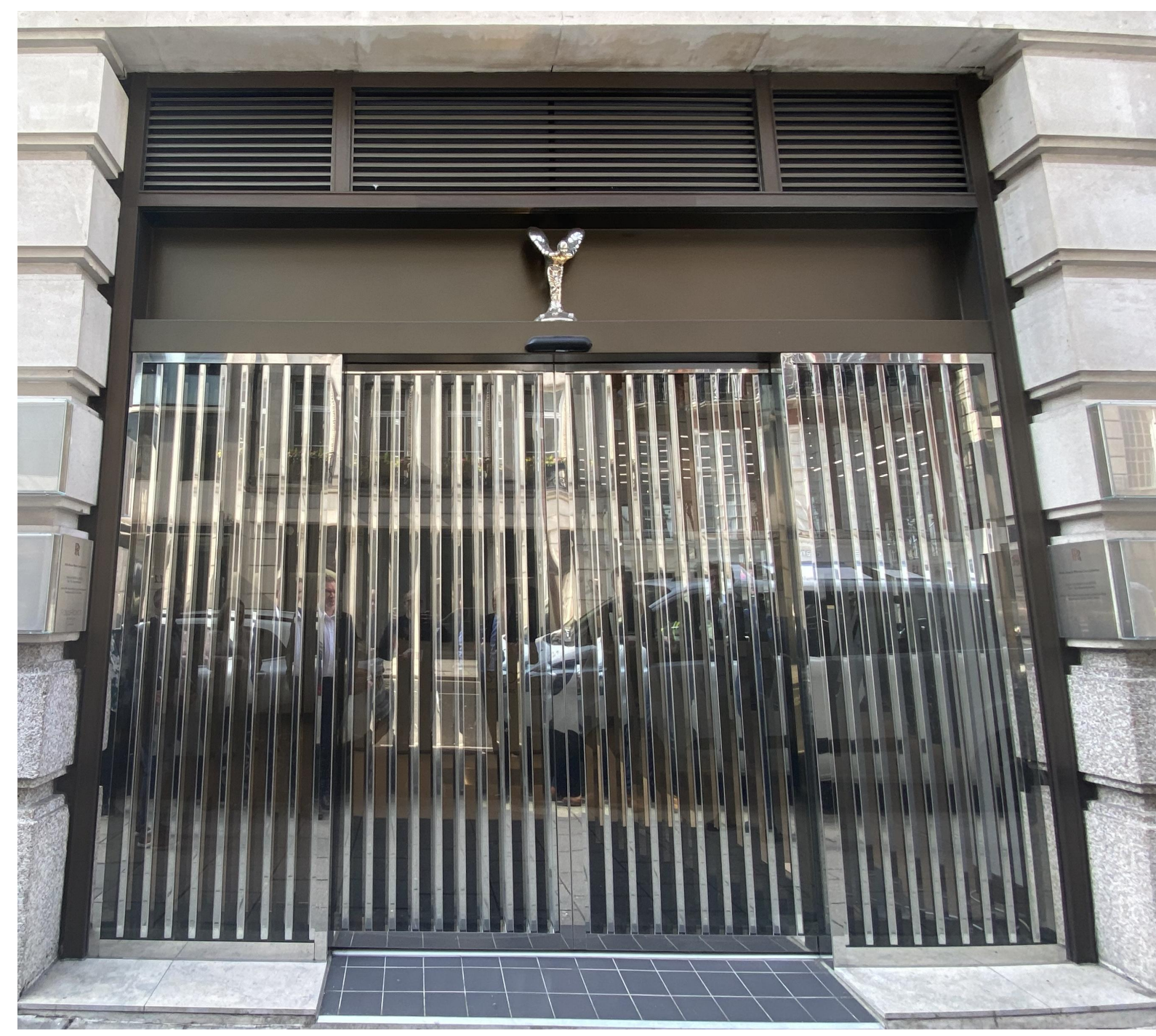
CHROME AND GLASS ENTRY DOOR ABOVE DOOR HEADER IS POWDER COATED STEEL (RAL 000 55 00)
