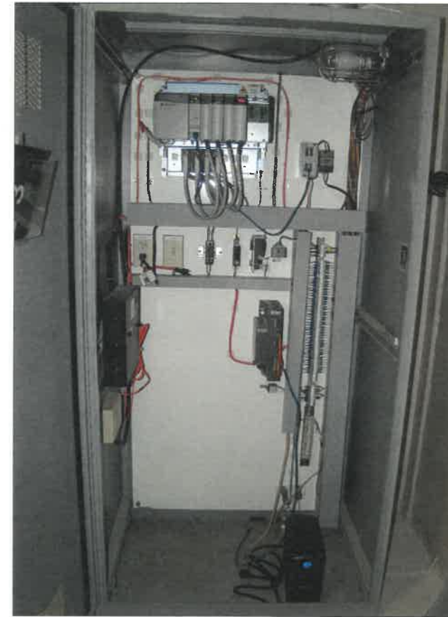
EX. MCC PLC CONTROL PANEL UNIFORM BLDG.
