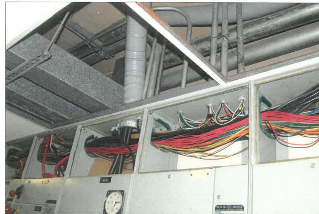
EX MCC-3 INCOMING TOP-ENTRY FEEDER UNIFORM BLDG.
