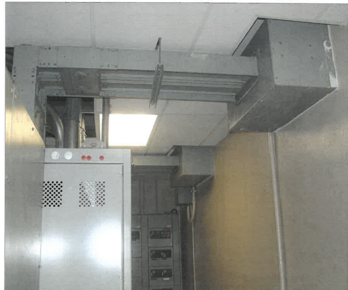
EX. SWITCHGEAR BUS DUCT TO FPL VAULT ELECTRICAL ROOM #1
