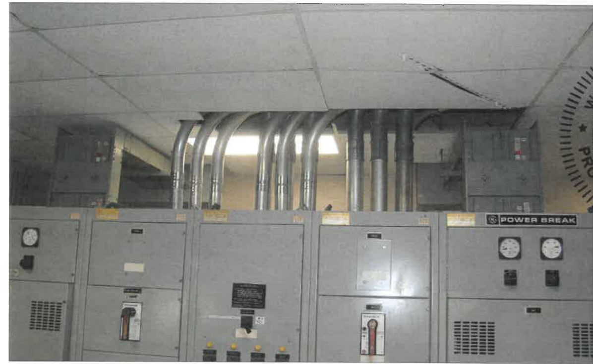
EX. SWITCHGEAR OVERHEAD CONDUIT AND BUS DUCT ELECTRICAL ROOM #1
