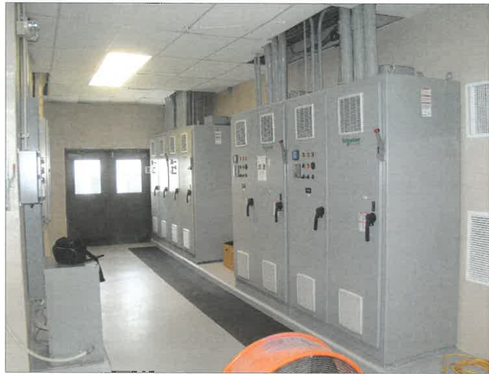
ERP-1,2 VFD'S AND ERP-3,4 VFD'S ELECTRICAL ROOM #1
