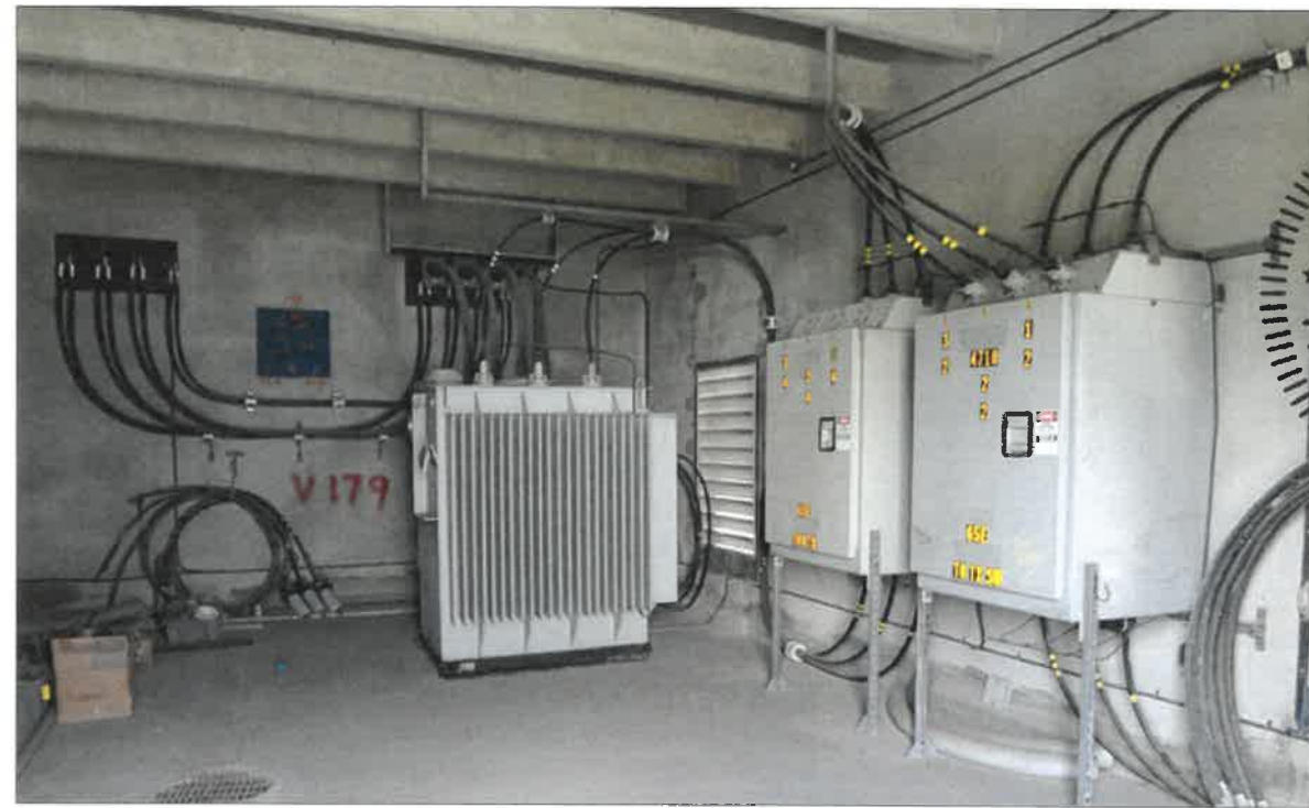
FPL VAULT ELECTRICAL ROOM #1
