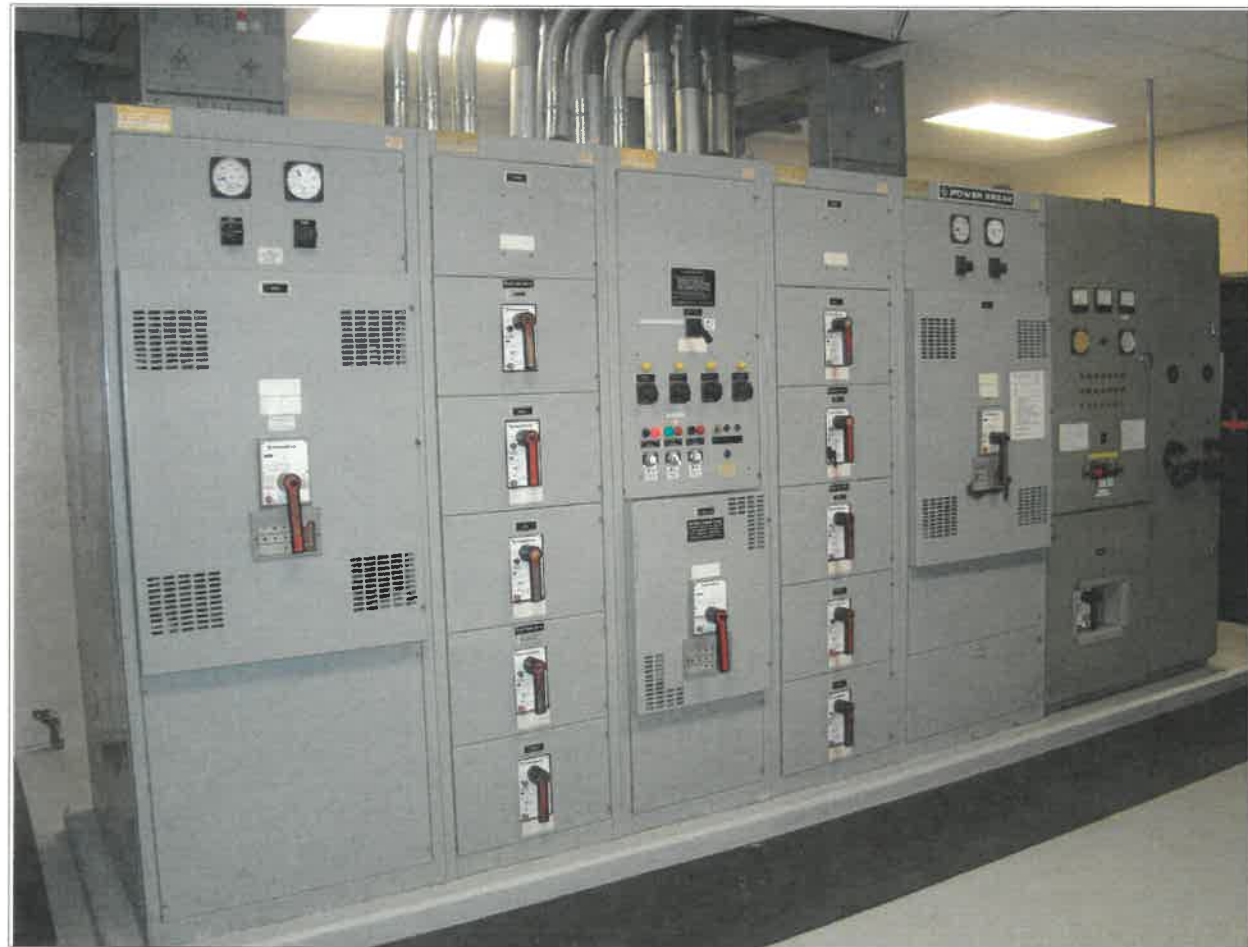
EX. SWITCHGEAR (FRONT VIEW) ELECTRICAL ROOM #1
