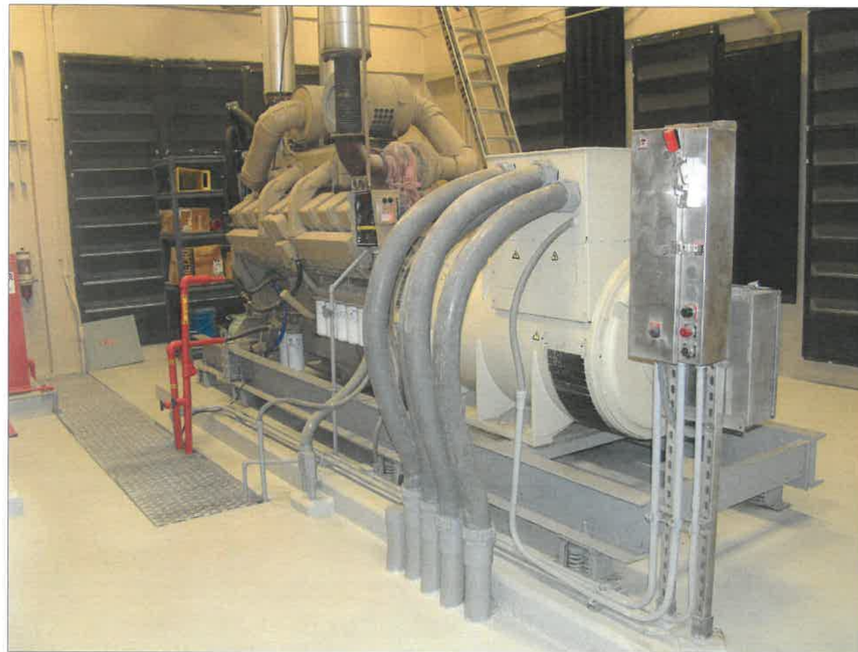
EX. GENERATOR #1 ELECTRICAL ROOM #1
