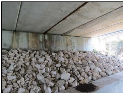
Undermining at End Bent 1
