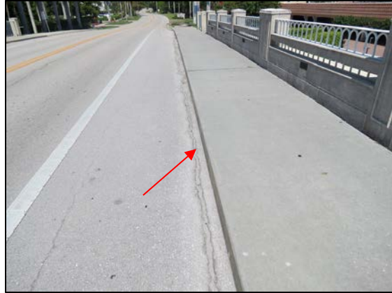
Typical cracks along curb lines (at widening joint)
