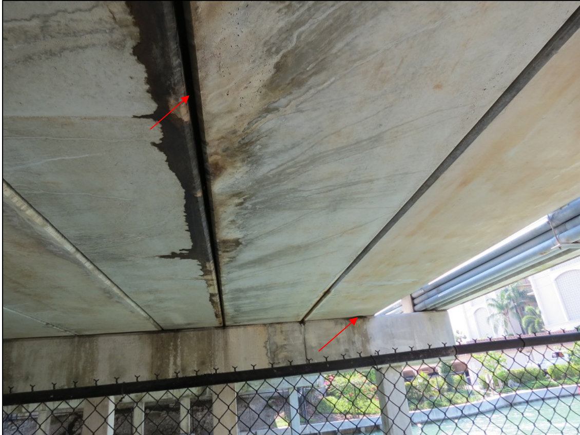
Minor spall at Slab Unit 1-12 and leakage through joints
