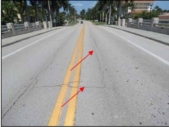
Typical condition of wearing surface
