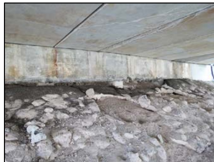
Undermining at End Bent 4
