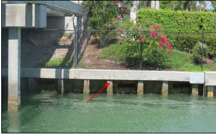
Seven piles at East sea wall (arrow on pile with spall)
