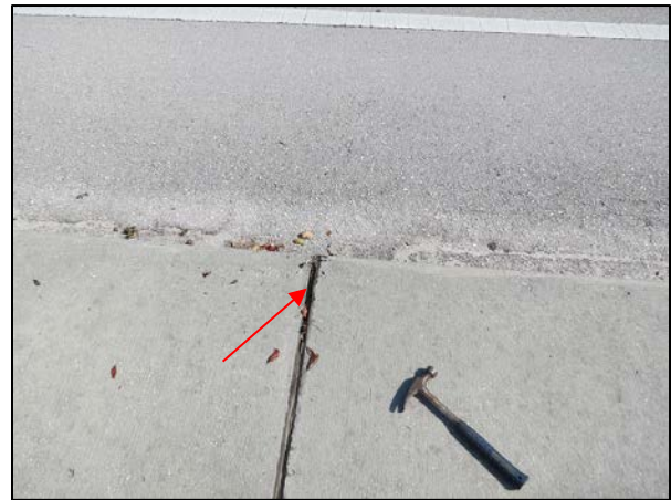
Adhesion failure (12" long) in sidewalk joint at Bent 3
