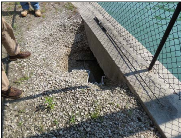
Sink hole on left side behind sea wall
