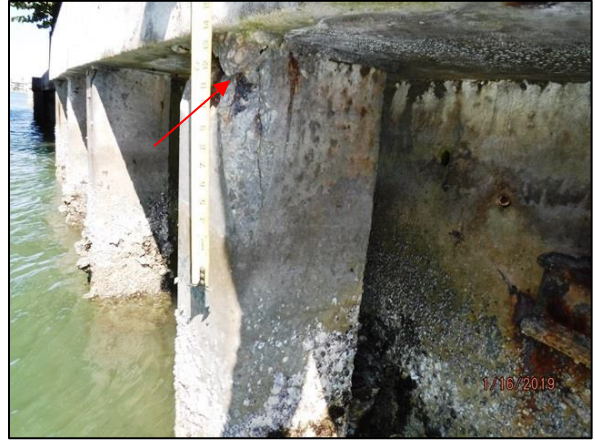
Close-up of pile spall and rusted channel
