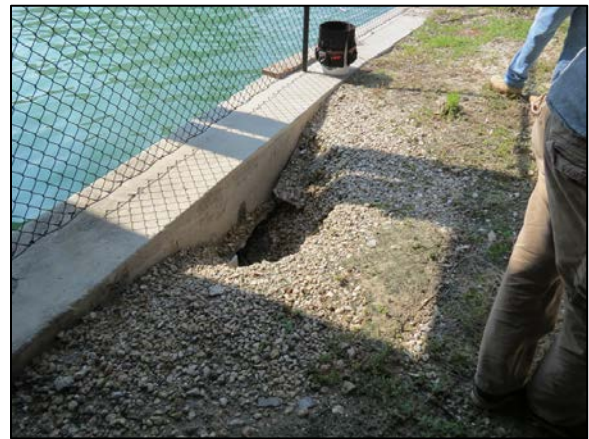
Sink hole on right side behind sea wall
