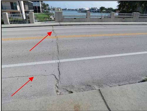
Pavement cracks at approach slab for End Bent 1
