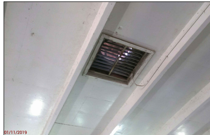
EXISTING ROOF TOP FAN – INTERIOR
