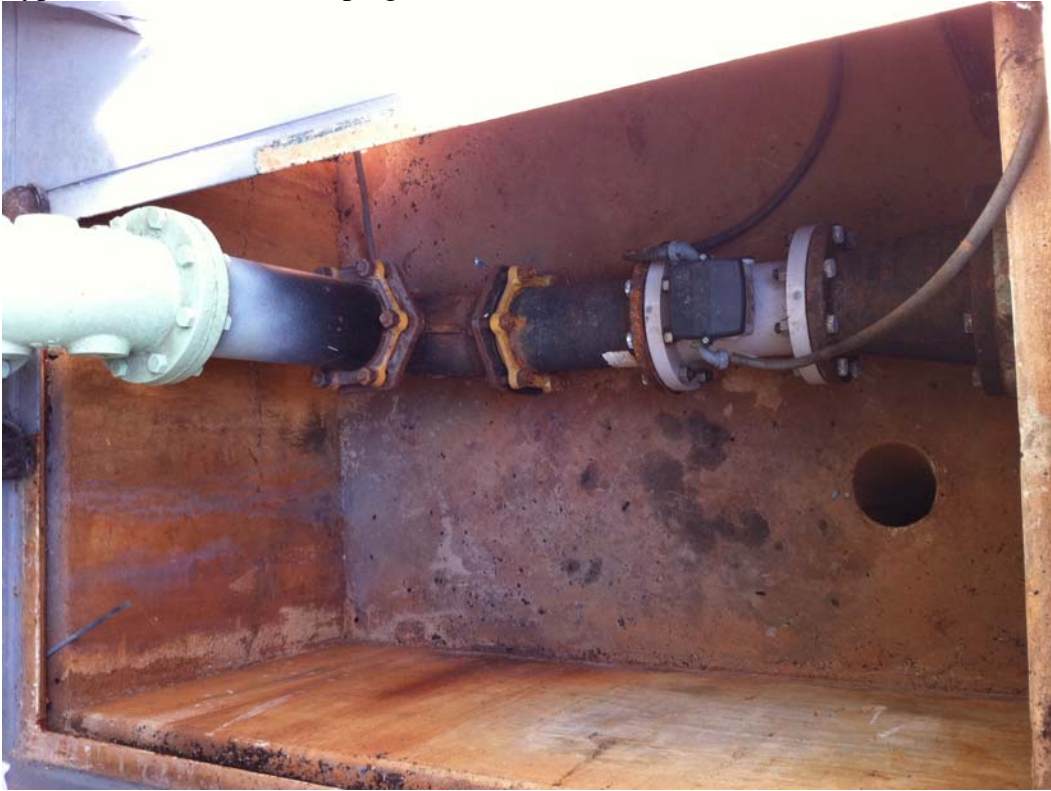
Typical Interior of Well Piping Vault:
